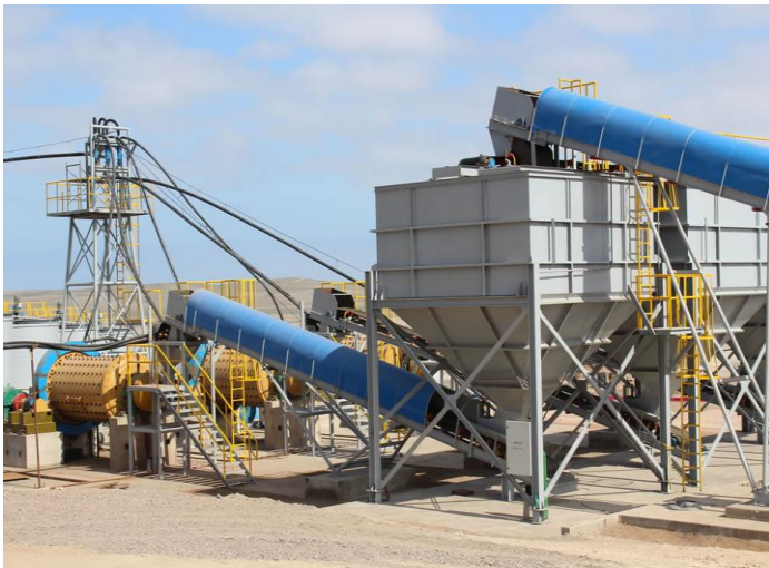
Kori One Plant crusher and ball mills circuit
